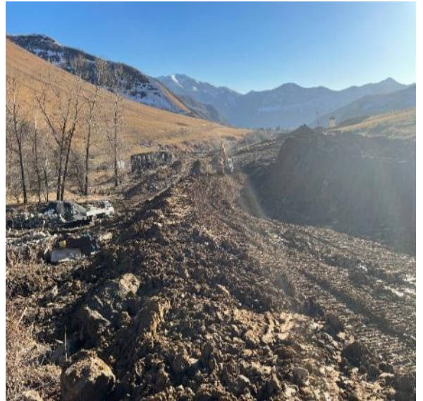
Access road to vil. Mughure which was several times improved by the Contractor
